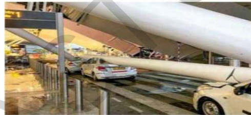
Crash impact: Vehicles crushed after a portion of the roof at the Delhi airport's Terminal 1 collapsed amid heavy rain on Friday. PTI
